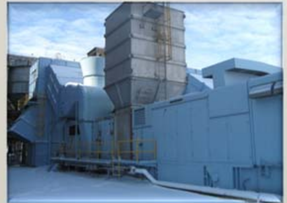
GE Gas turbine
