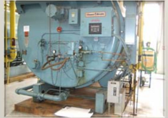
Cleaver Brooks boiler
